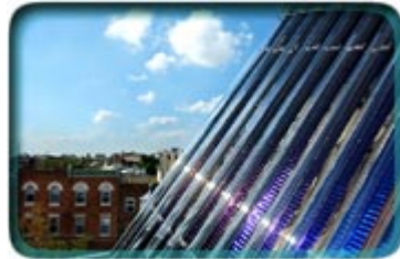
Sun Rah!: Solar panels on the roof of 1005 S. Seventh St. Photo By: Michael T. Regan
